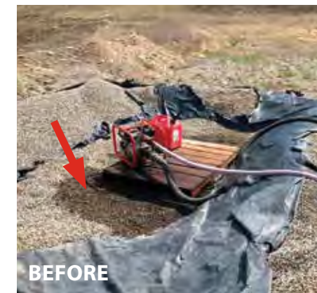
Gasoline spill before clean-up
