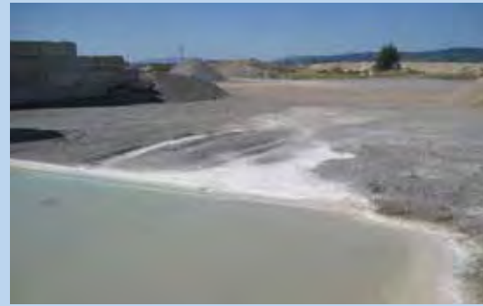
Overflowing truck washout basin at a concrete plant
