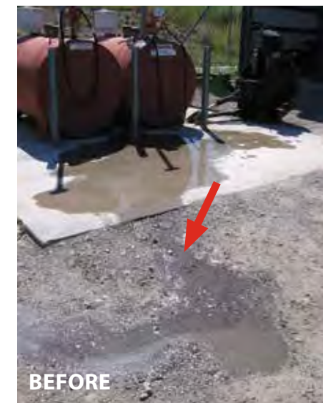
Uncovered, spills go off pad onto ground, no grit chamber/blind sump
